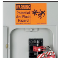
Safety Sign Labeling
