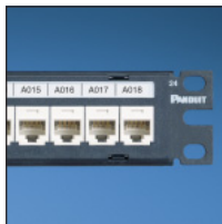
Patch Panel Labeling
